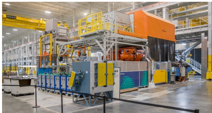
This modern die casting cell has an exhaust air volume of 20,000 m 3 /h and is equipped with its own KMA smoking hood and filter system
