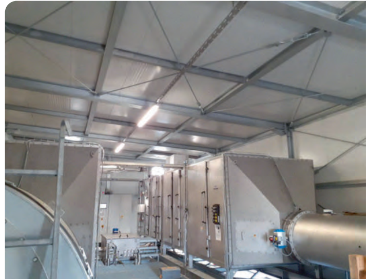
Two-filter systems for a total exhaust air volume of 60,000 m 3 clean the odour-laden exhaust air and recover process waste heat. Photo: KMA Umwelttechnik
