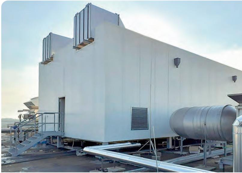
The central filter system is located in the weather protection housing on the roof. Photo: KMA Umwelttechnik
