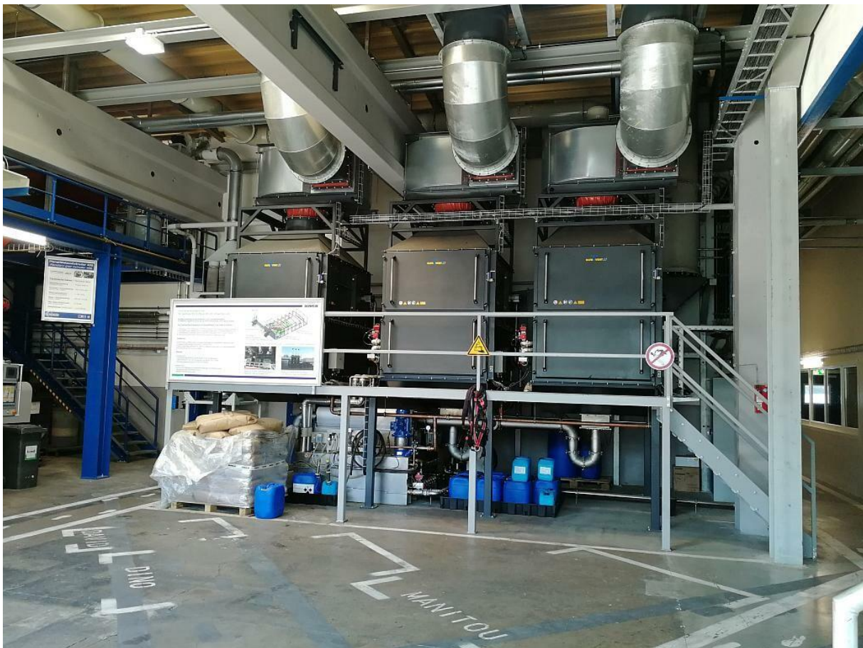
The electrostatic filter modules with integrated heat recovery and CIP washing system ensure high efficiency. (Fig.: KMA)
