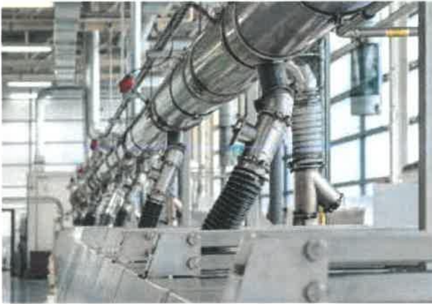
The exhaust air is extracted at several points above the salt bath vulcanisation system.
